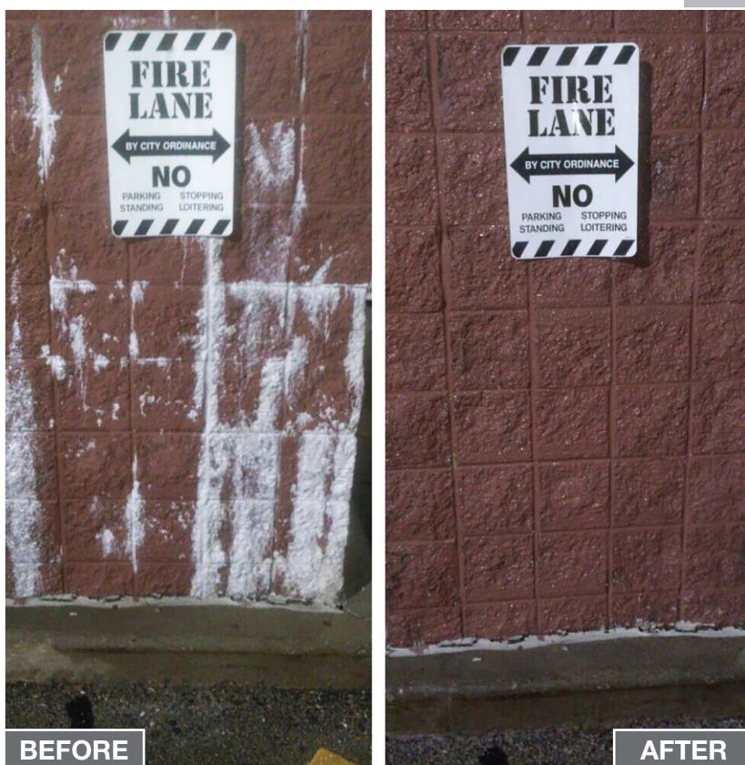
Efflo Process #1 Powdery Efflorescence
