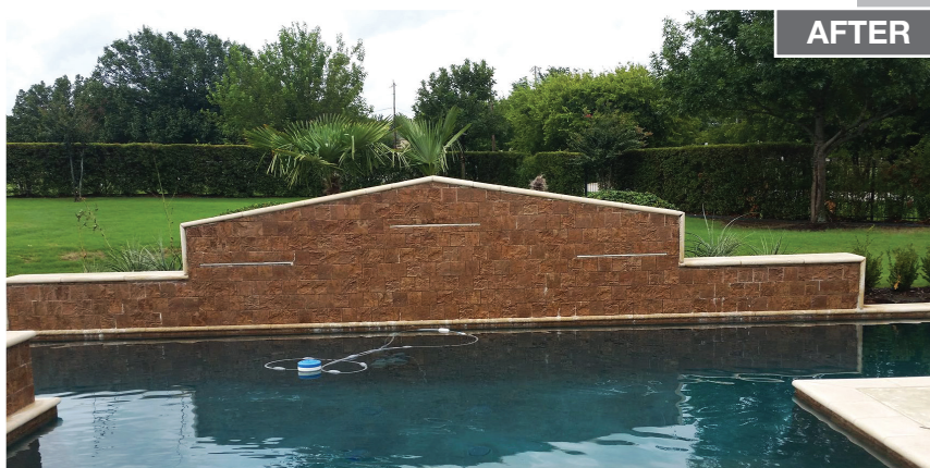
Efflo Process #2 Calcium Carbonate and Lime Run on Porous Brick Patriot Services Bedford, TX
