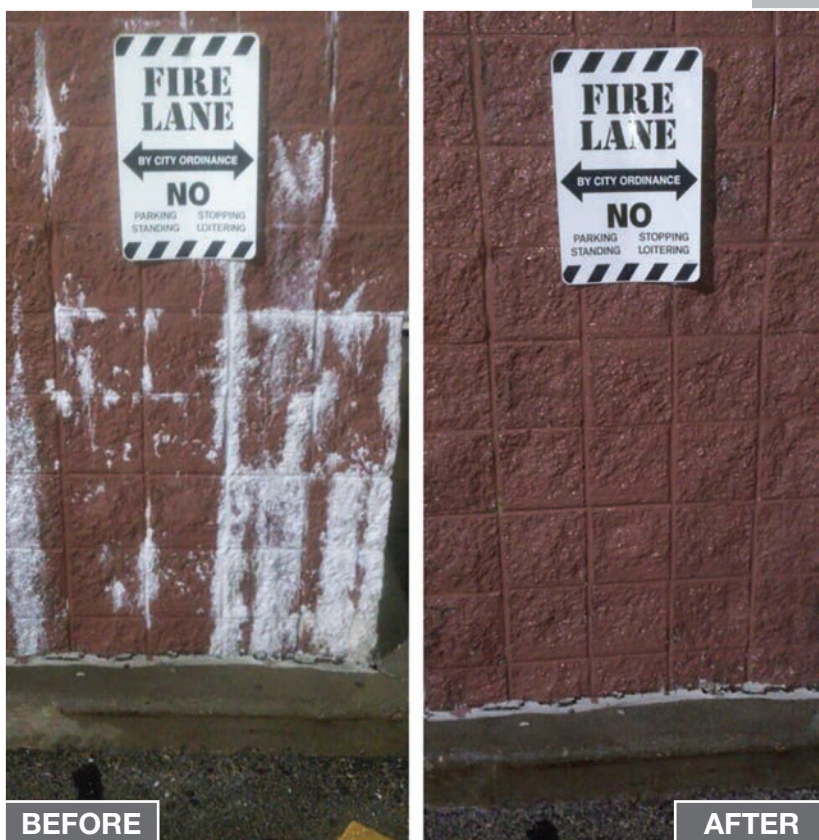
Efflo Process #1 Powdery Efflorescence
