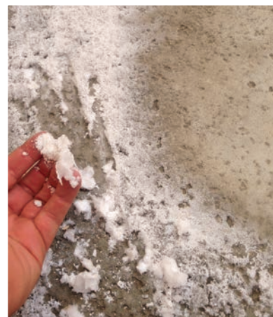
Use Efflo Process #1 Powdery Efflorescence on Concrete Eco Friendly Power Washing Palm Desert, CA
