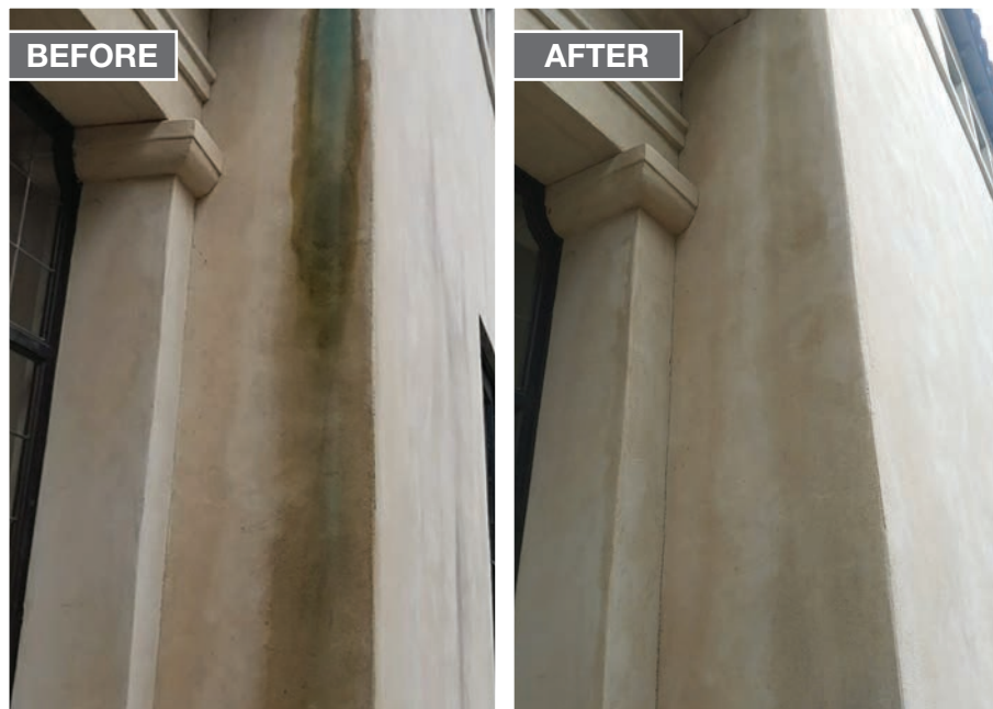
Efflo Process #2 Copper Stains on Stucco Squeaky Dan's LLC San Antonio, TX
