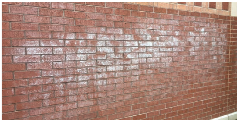
Efflo Process #1 Powdery Efflorescence Clean and Green Solutions Houston, TX
