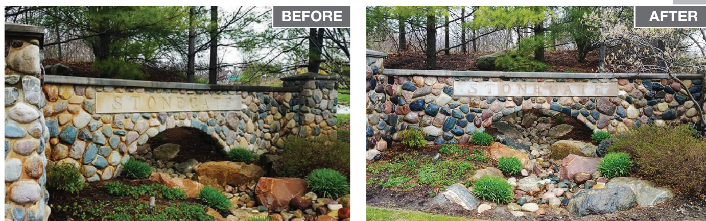
BARC Process #1 Light Rust Stains on Stone
