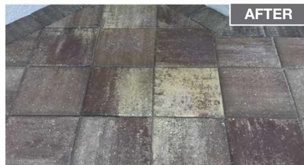
BARC Process #1 Heavy Rust and Fertilizer Rust Stains Spray Soft Exterior Cleaning Smyrna Beach, FL
