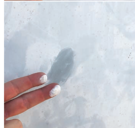
Painted surface oxidation
