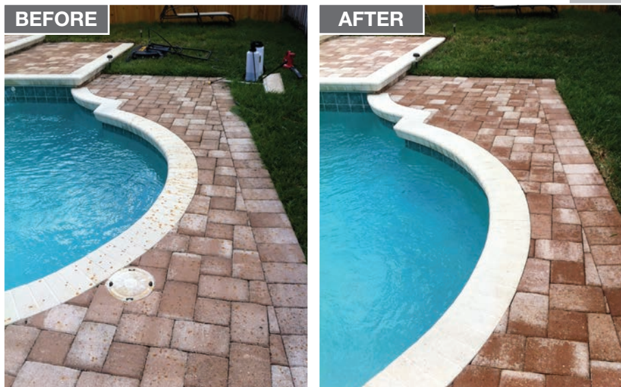
BARC Process #1 Fertilizer Rust Stains on Pavers
