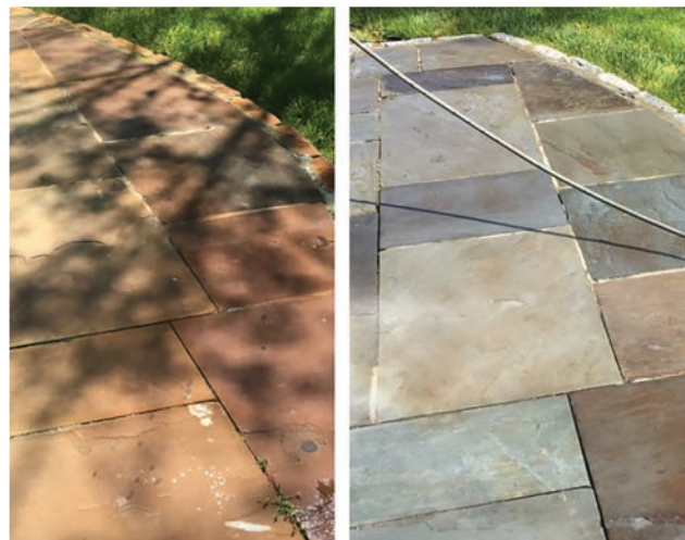
BARC Process #2 Irrigation Rust Stains on Tile
