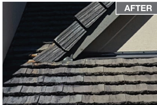
Rust on Cedar Shake Shingle
